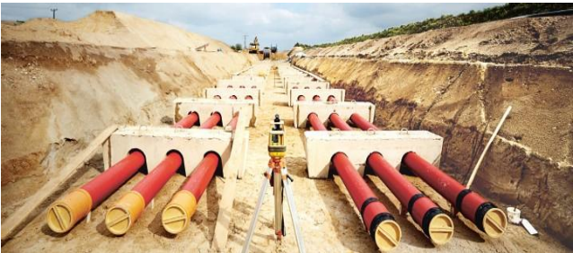
Pipes for power grids
